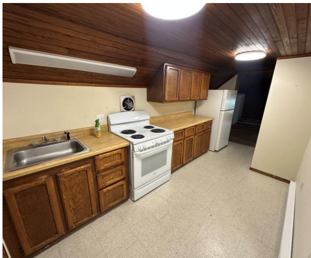
3 rd Floor Kitchen
