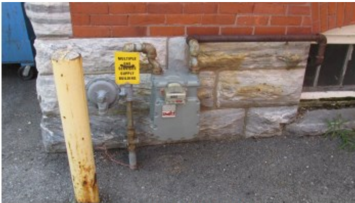
GAS SUPPLY ENTRANCE
