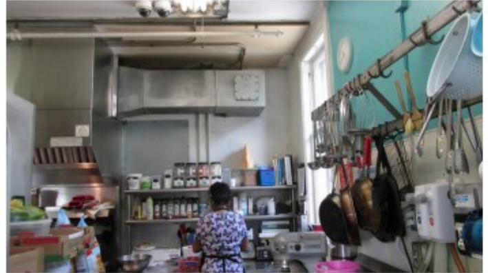
KITCHEN EXHAUST INTERIOR
